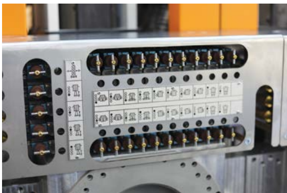
Valve block for cooling only valves.
